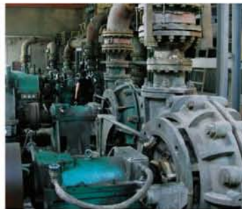
两台 150ZGB 高扬程渣浆泵串联， 输送浓缩和底流煤浆。 Two 150ZGB high head slurry pumps in series pumping coal tailings direct from a thickener underflow.
