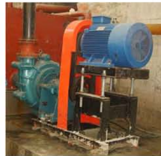
SH/150E渣浆泵在洗煤厂的应用。 A SH/150E slurry pump delivering fine coal to dewatering screen in a coal washery.
